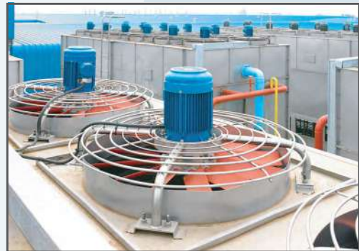
Fan and water pump
